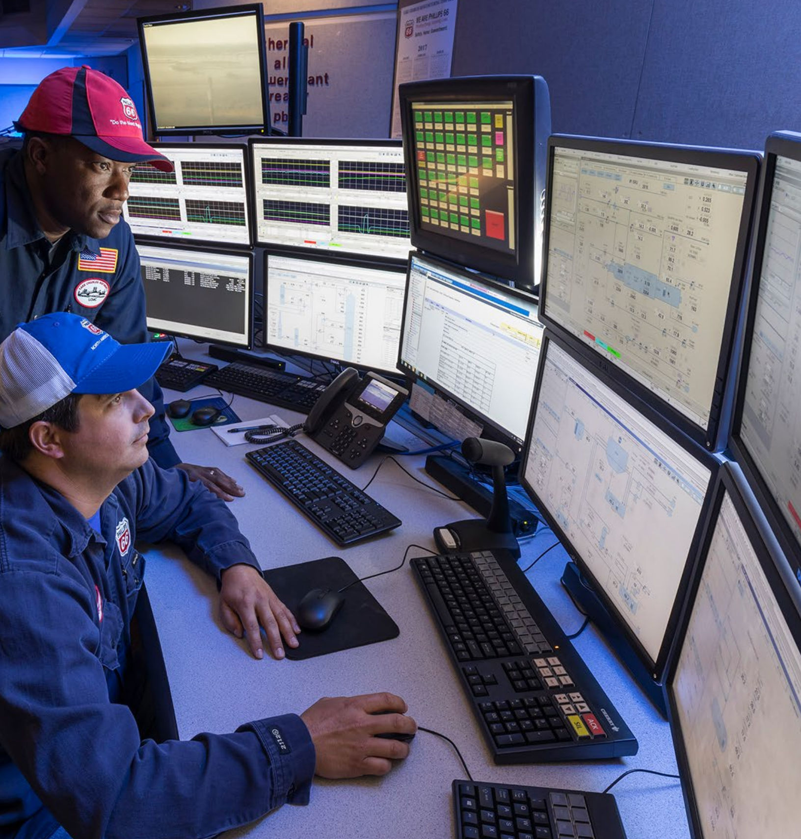
PHILIPS 66 CONTROL ROOM Louisiana
